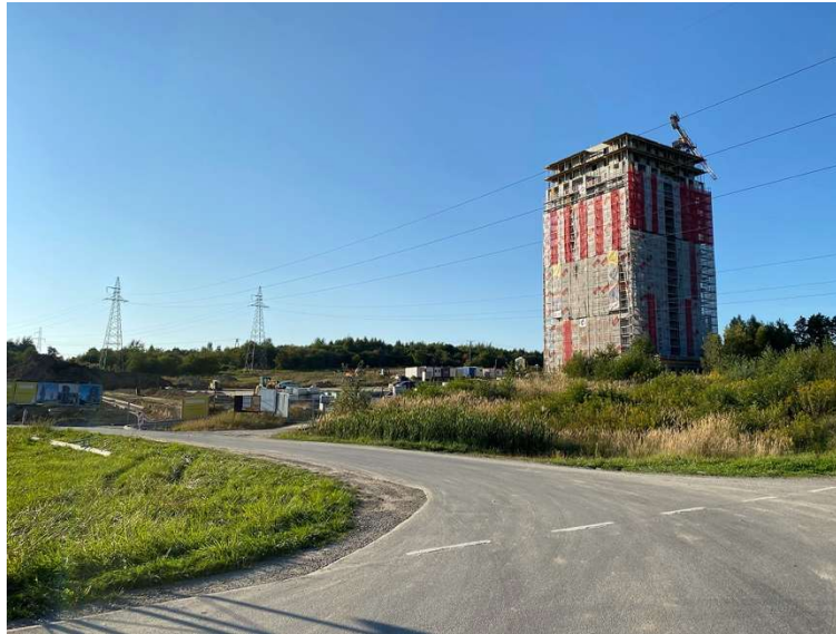
Fig. 5. View of the first high-rise building of the Carpatia housing complex that is being constructed. Photo by J. Figurska-Dudek
