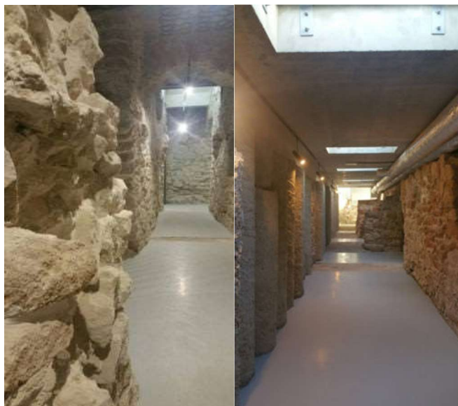
Fig. 18. Cellars after uncovering and renovation. Palisade retaining wall (on the right) (Photo by the author)
