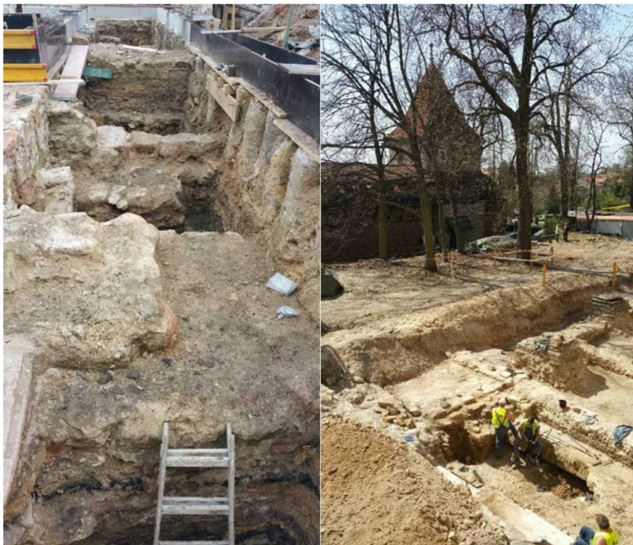
Fig. 11. Archaeological research and gradual uncovering of buried, medieval cellars under the courtyard (Photo by the author)
