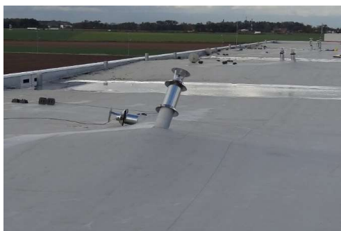
Fig. 4. Damage to the roof of the hall no. 1. Overturned roof ventilation chimneys
