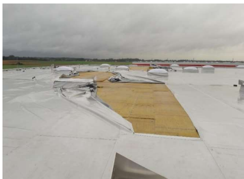
Fig. 5. Damage to the roof of the hall no. 2. A detached membrane in the perimeter zone, exposed thermal insulation
