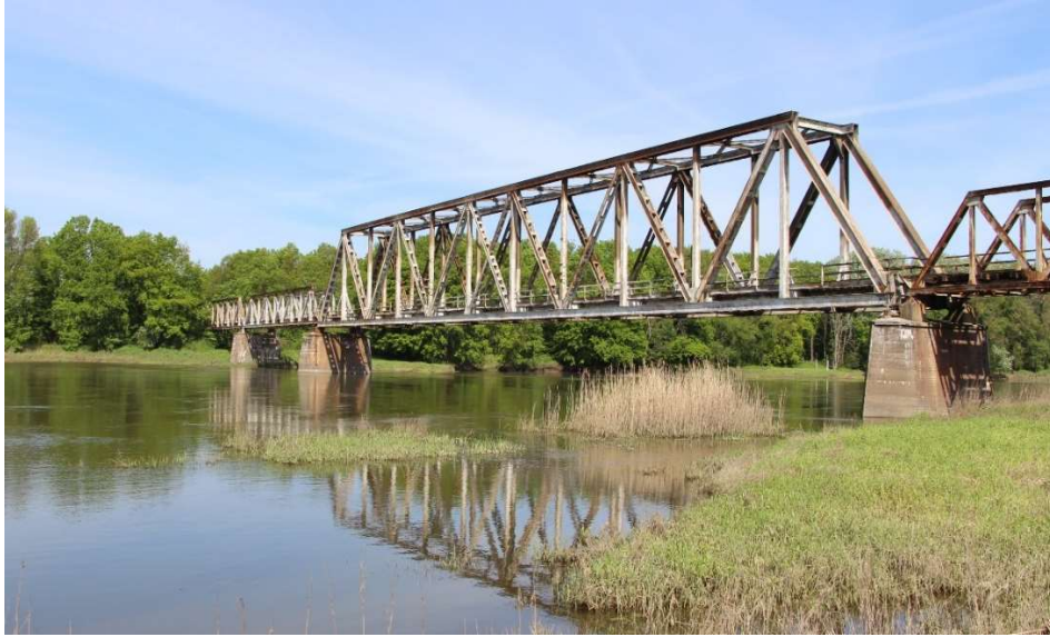
Fig. 7. Parallel lattice of the river span, a view from the western side (photo by the Author, 2017)
