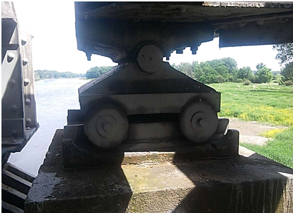
Fig. 8. Steel sliding bearing (photo by the Author, 2012)
