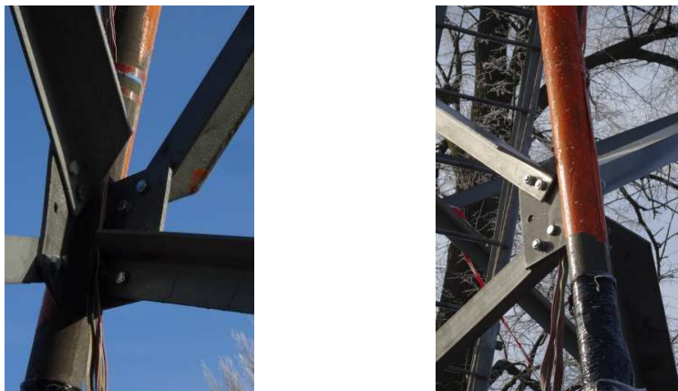
Fig. 4. Deformed gusset plates in middle span of the leg in the lowest section.
