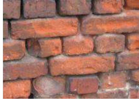
Fig. 4. The effects of corrosion in the wall on lime mortar of lower strength than brick
