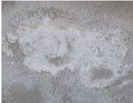
Fig. 1. Surface crystallization-wall and plaster remain overdamped
