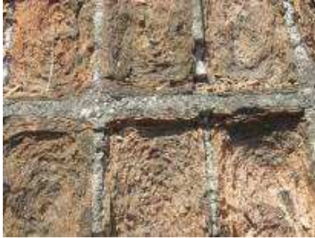
Fig. 3. Effects of corrosion with cement mortar stronger than ceramic material
