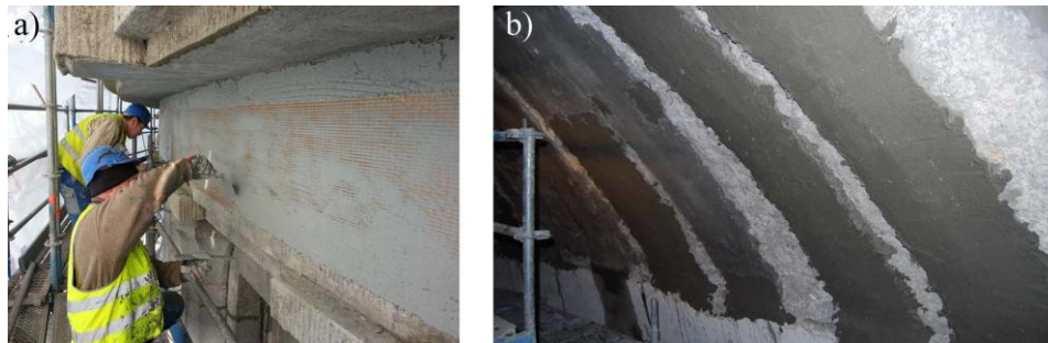
Fig. 1. a) Reinforcing the support ring using P.B.O. fiber mesh; b) Reinforcing the shell from the inside using carbon mesh
