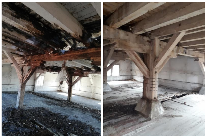
Fig. 5. Structural elements damaged by fire, uncontaminated section of building structure author archive
