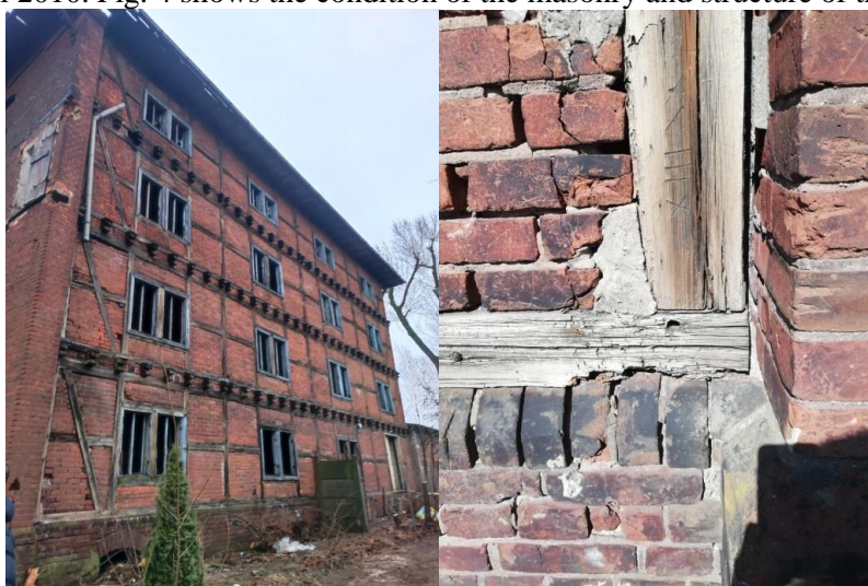
Fig. 4. Elevation of the retrofitted building, condition of the masonry samples author archive
