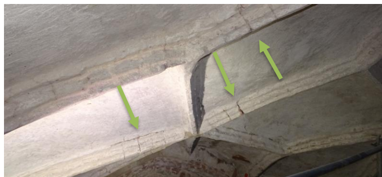
Fig. 26. Cracked ribs in rib vaults in St. John's Church in Malbork
