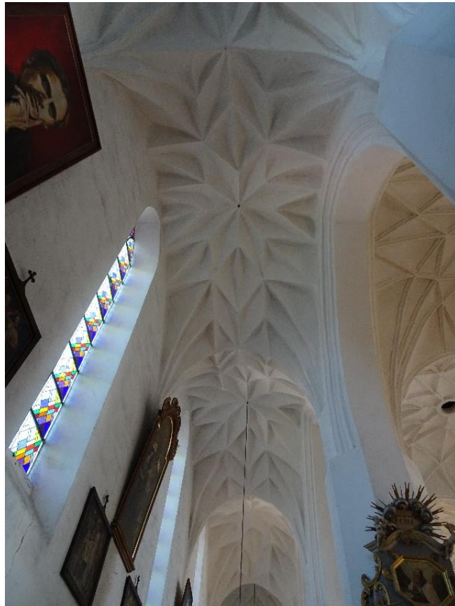
Fig. 10. Diamond vaults over the chapel in St. Anne and Stephen's Church in Barczewo
