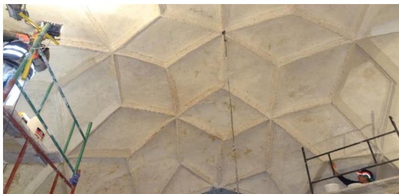
Fig. 28. Restoration works performed underneath the rib vaults in St. John's Church in Malbork
