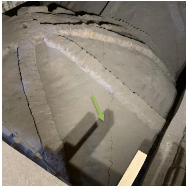
Fig. 25. Crack in rib vaults in St. John's Church in Malbork (photo by M. Jackiewicz)
