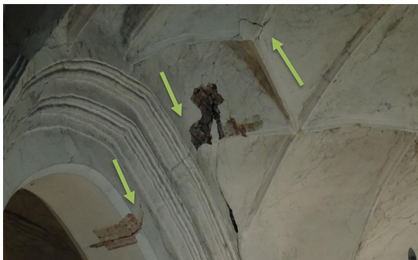
Fig. 24. Cracks in rib vaults in St. John's Church in Malbork
