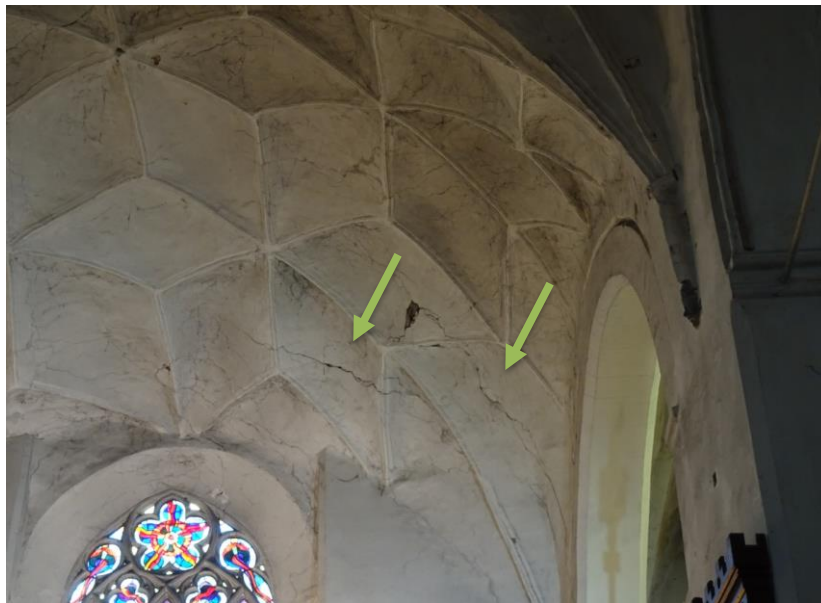
Fig. 23. Cracks in diamond vaults in St. John's Church in Malbork
