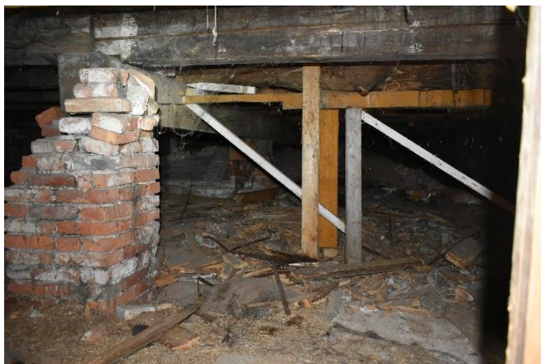
Photo 10. Damage to the ceiling and its supports – pillars
