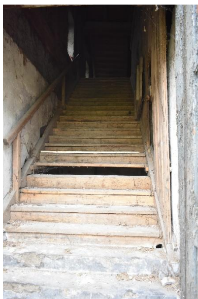
Photo 9. Damaged wooden stairs
