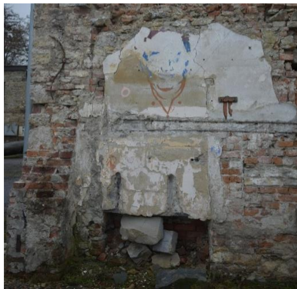
Photo 3. Damage to the western corner of the Kossak Manor Granary
