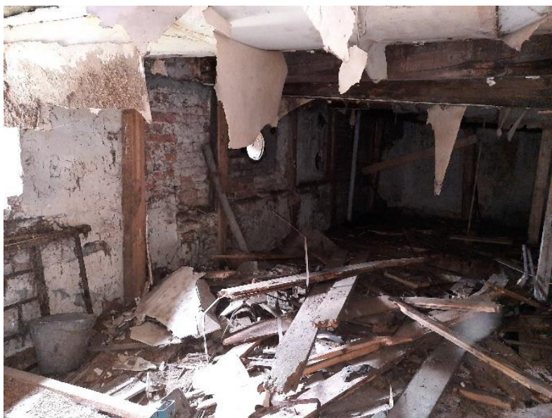
Photo 8. Damaged wooden ceiling
