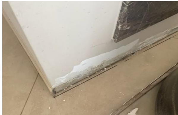
Fig. 6. Level of water ingress inside the building
