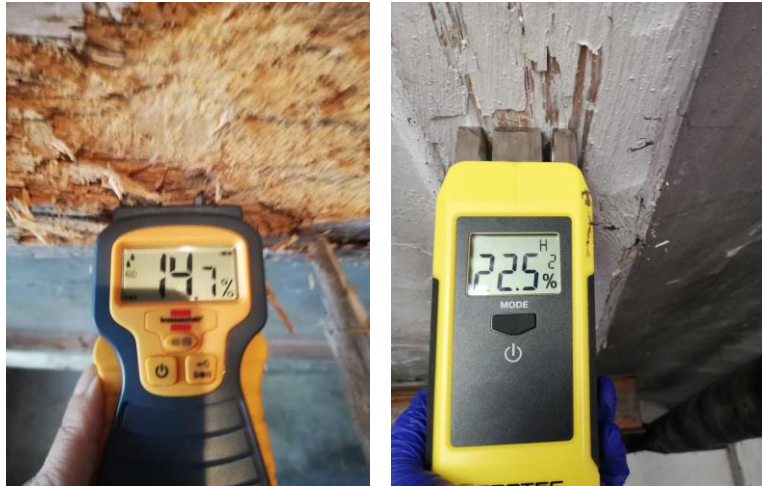
Fig. 3. Moisture measurements of a flooded structure 2 years after failure
