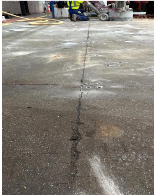
Fig. 2. Degraded concrete industrial floor (Example 1): visible wear of the top layer, mounting anchors left over from equipment removal, and shrinkage joint damage [38]
