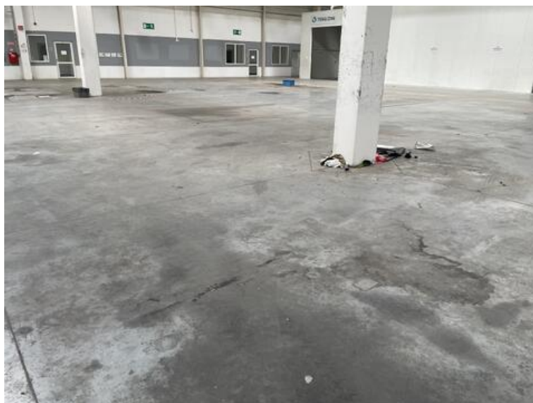
Fig. 14. Concrete industrial floor (Example 4) before renovation: damaged upper floor surface due to improper use of cleaning agents [38]
