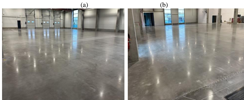
Fig. 13. Concrete industrial floor (Example 3) after regeneration by polishing and impregnation process: a) general view, b) view of pavement treatment in the area of structural expansion joints [38]
