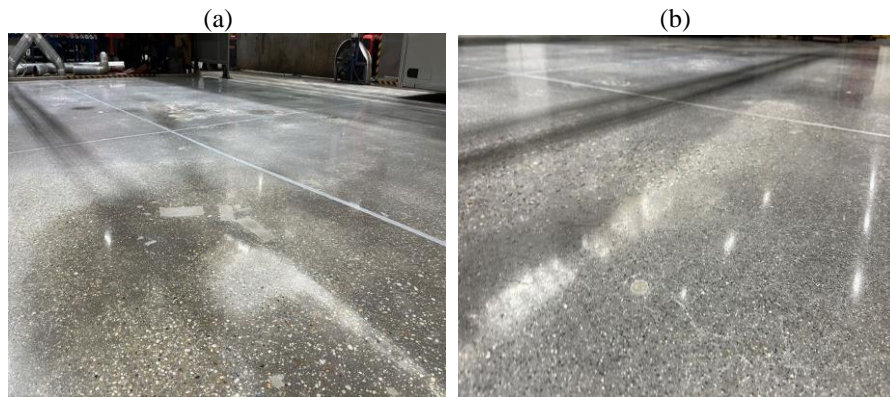
Fig. 8. Concrete industrial floor (Example 1) after repair: a) visible areas of repair of cavities b) visible areas of repair after anchors [38]
