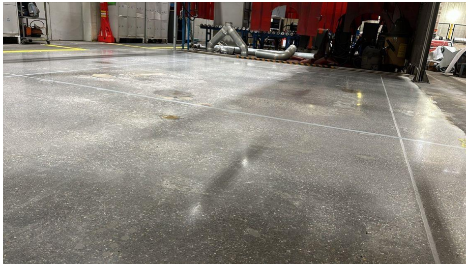
Fig. 9. Concrete industrial floor (Example 1) after repair: general view and visible reconstructed and completed shrinkage expansion joints [38]
