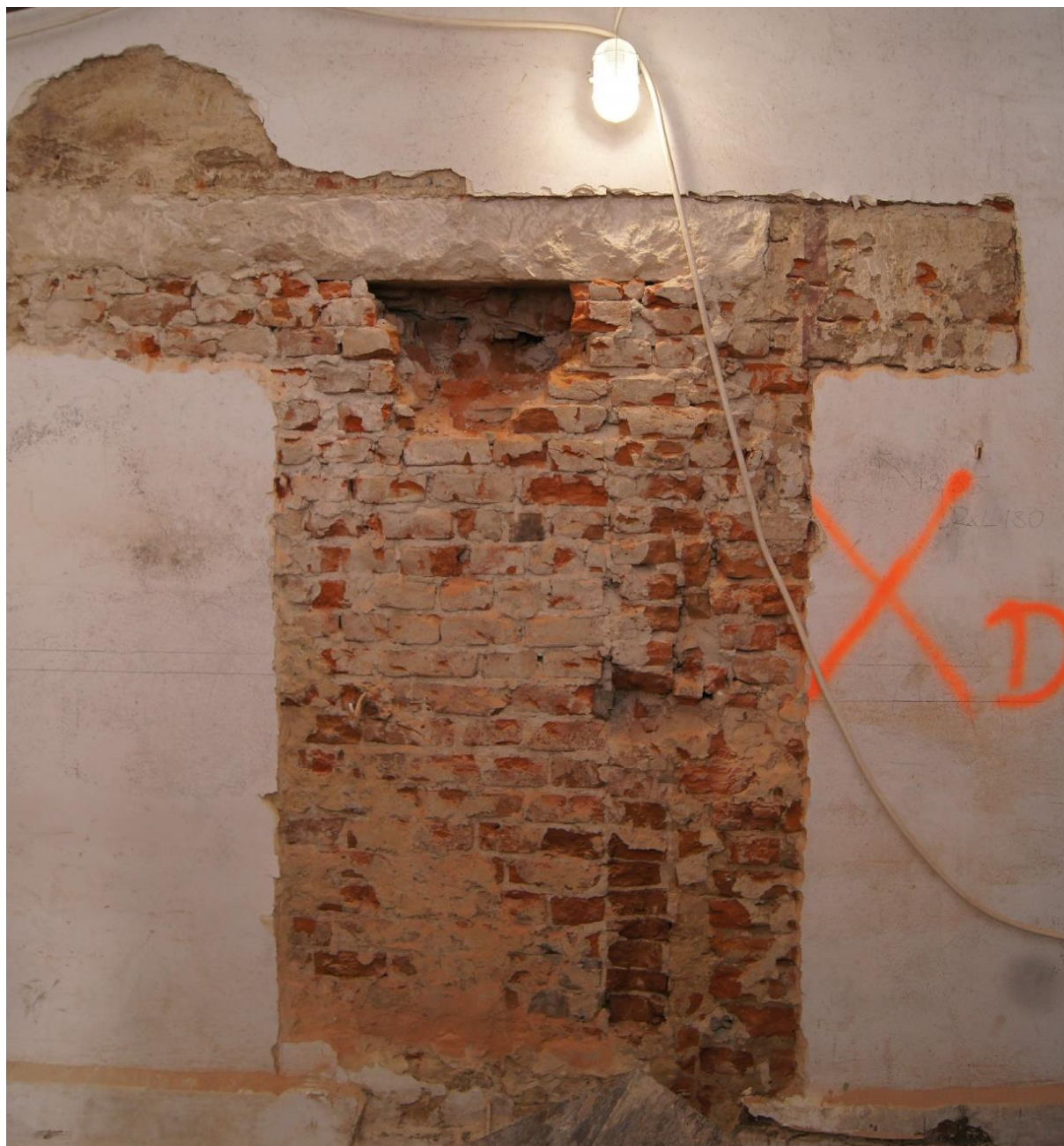
Fig. 10. Remains of the stone lintel beam, photo by K. Janus, 2024
