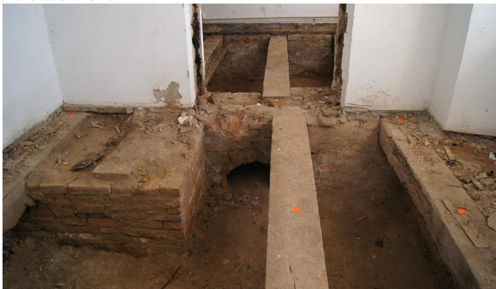
Fig. 3. Visible ventilation opening between the rooms of the ventilated floor and the beams/joists of the floor, photo by K. Janus, 2021
