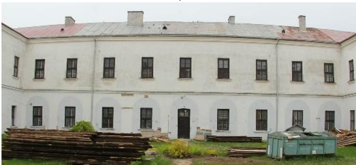
Fig. 6. View of the academy courtyard from the east before the renovation began, photo by K. Janus, 2021
