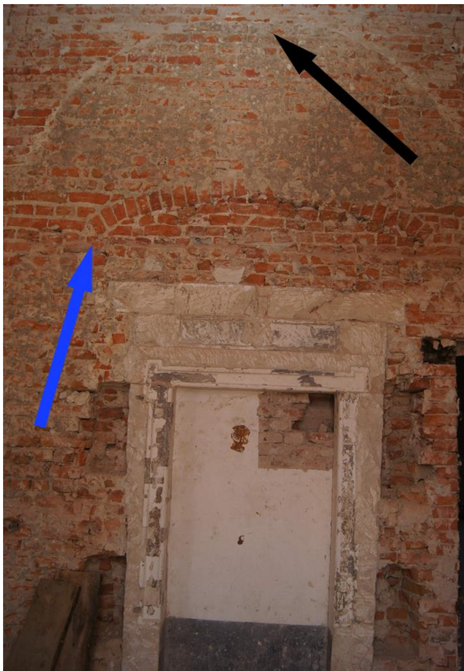
Fig. 11. Damaged stone portal with a visible relieving arch (blue arrow) and the negative of the vault (black arrow), photo by K. Janus, 2021
