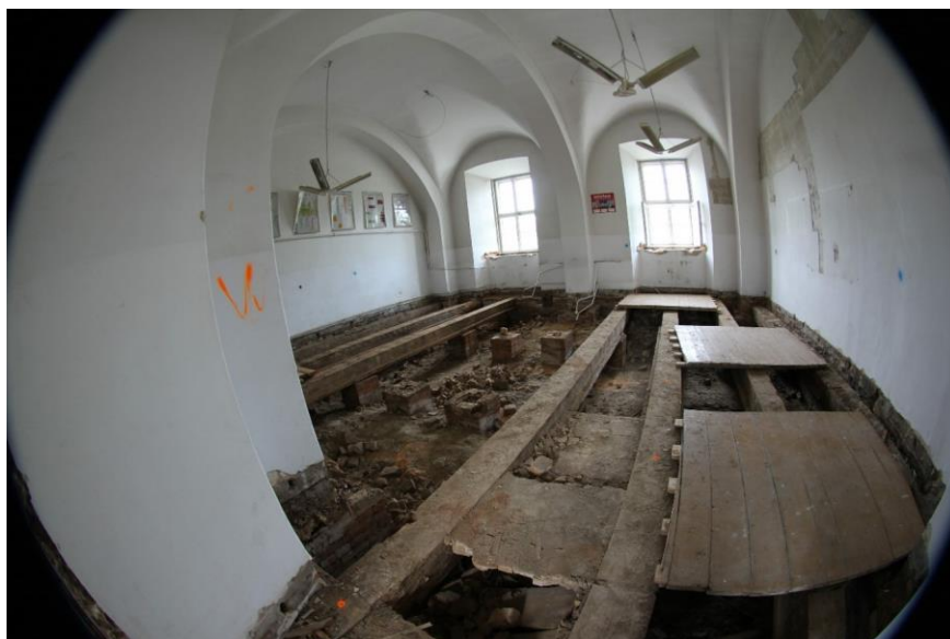
Fig. 20. Kanty's Room before the start of conservation work, showing the ventilated floor, photo by K. Janus, 2021
