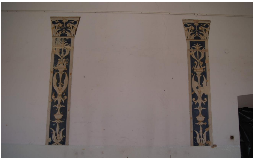
Fig. 26. One of the walls of the former library with fragments of interwar polychromy, photo by K. Janus, 2021
