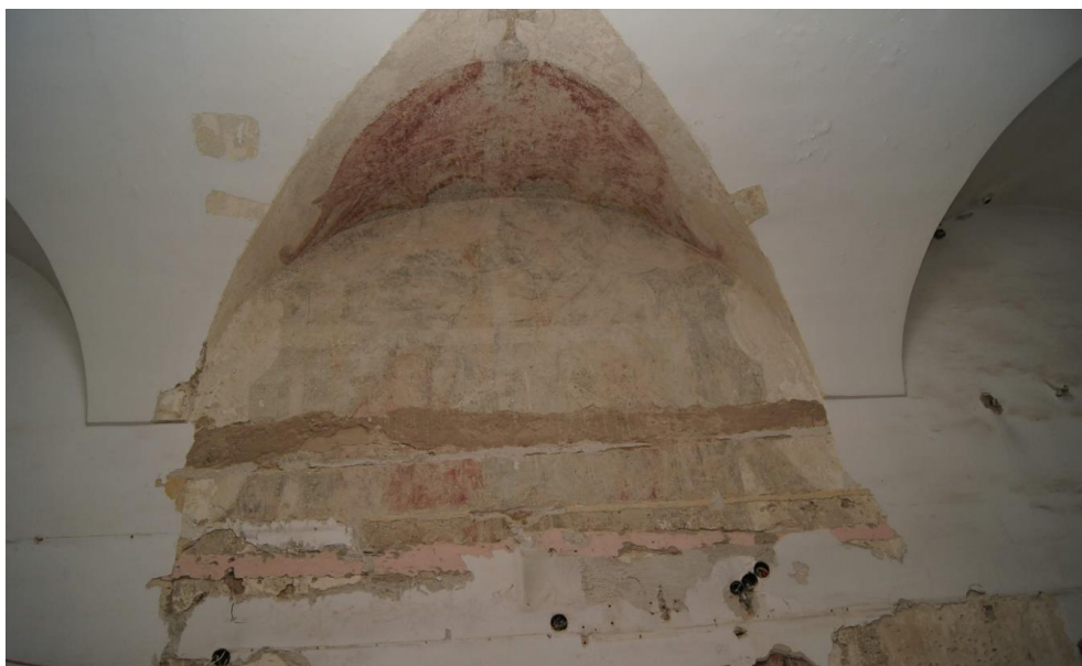
Fig. 24. Entrance to the former chapel during conservation works, photo by K. Janus, 2021
