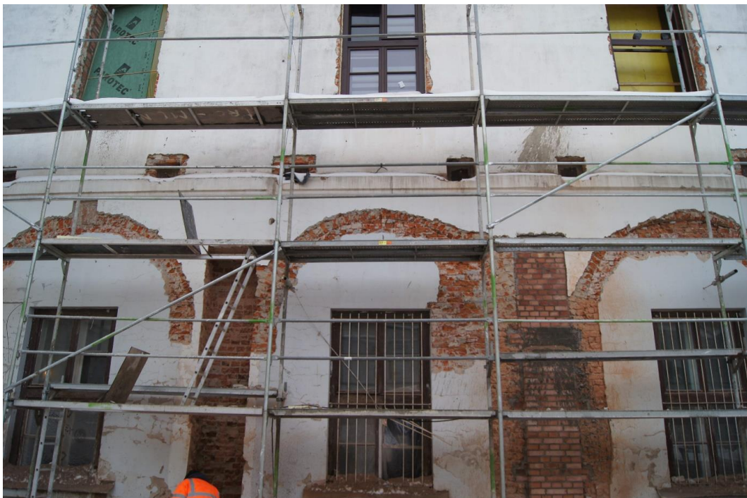
Fig. 5. Arcades during reconstruction, with the red arrow indicating the locations of the grooves for wall reinforcement, photo by K. Janus, 2022
