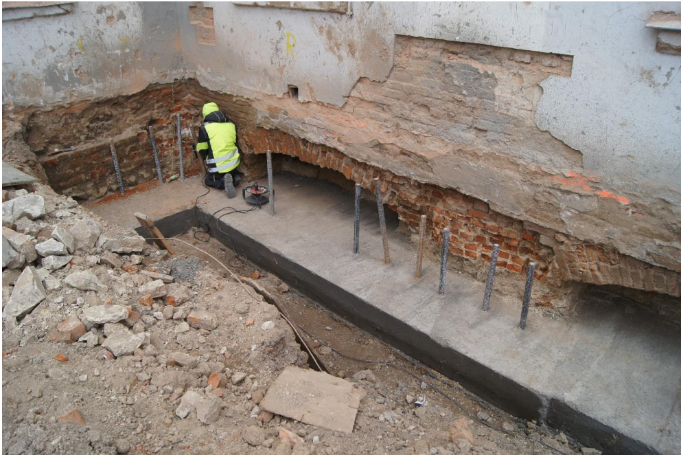
Fig. 4. North-East corner of the courtyard with visible original point foundations and brick arch during reinforcement works on micropiles, photo by K. Janus, 2023
