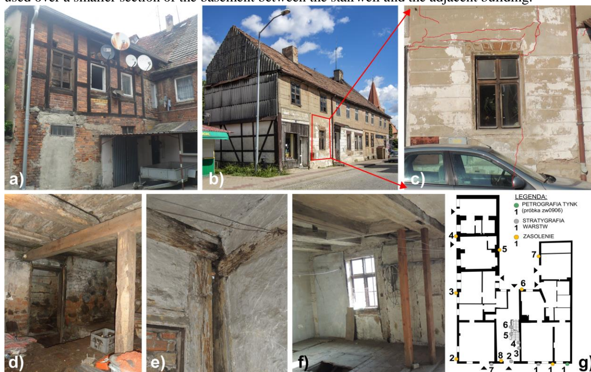
Fig. 4. Condition of the Building's Structural Elements: a) Northern Wing annex– Visible Deformations of the Timber Frame Structure, Secondary White Window Joinery, b - c) Southern Wing annex – Cracked, Moist, and Discolored (Salt-Damaged) Exterior Plaster, Secondary Asbestos Sheet Finish on the Gable, Secondary Extension Adjacent to the Internal Stairs Leading to the Basement (Marked with a Red Arrow ), d) Main Building Basement – Moist Stone-Brick Walls, Wooden Ceiling with Visible Signs of Insect Infestation, e) Ground Floor of the Southern Annex – Separation of the Timber-Framed Wall Construction, f) First Floor of the Northern Annex – Emergency Shoring of the Wooden Ceiling with Props, g) Ground Floor Plan – Sample Collection Points for Analysis. Source: Author's Documentation and Photos
